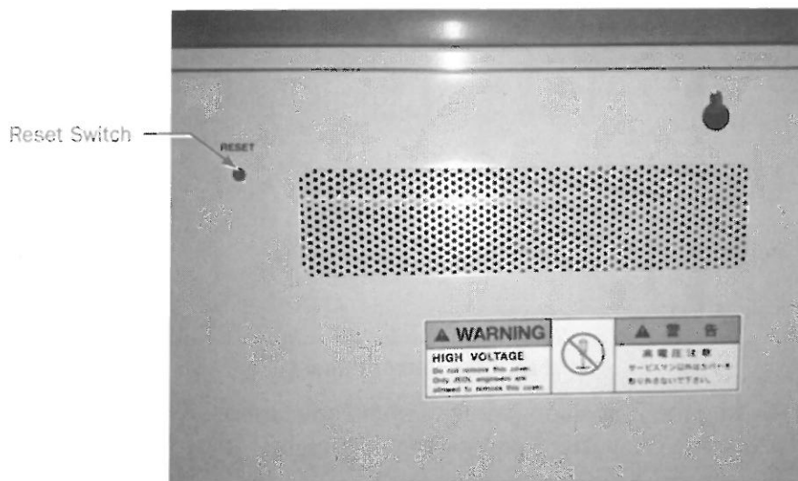
Fig. 4.8 Control Panel RS
